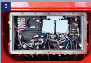
Electrical control system
